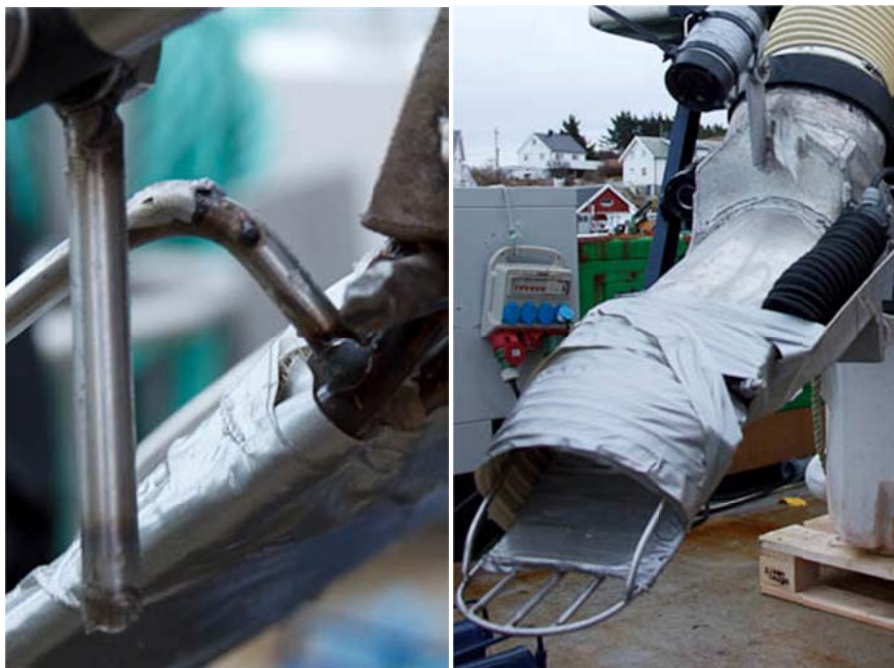
Figure 7 Broken welding and repair (second modification in Trial 1).
